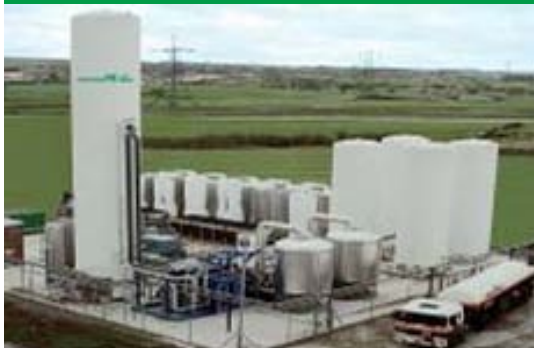
Onsite Gas Supply
